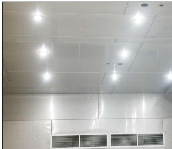
Figure 24: Explosion Resistant Interior Lighting
