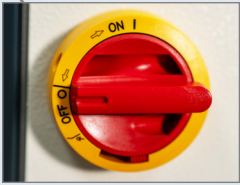
Main Power Switch
